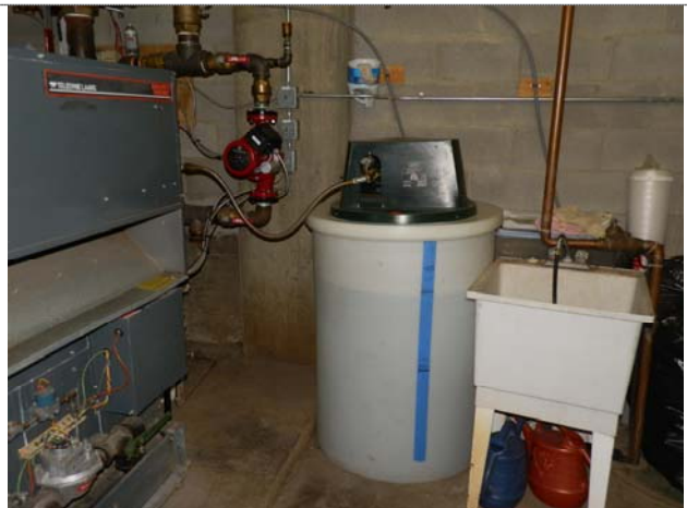
Axiom system feeder
