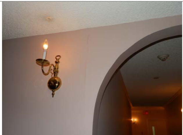
Cracking in wall finish
