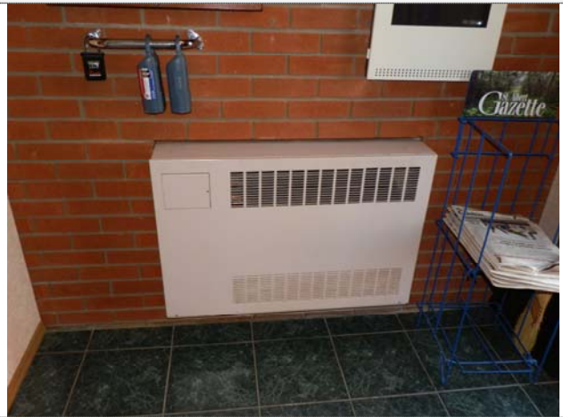
Cabinet heater at entrance
