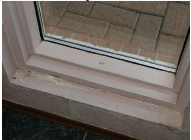
Damaged interior sill of sealed window
