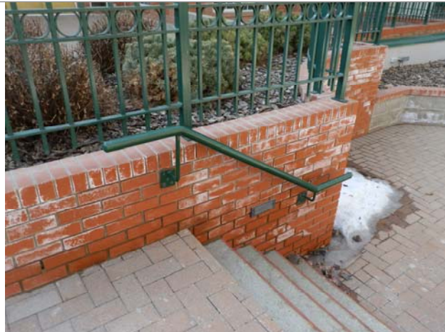
Brick walls with efflorescence
