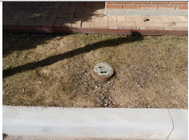
Shut off valve
