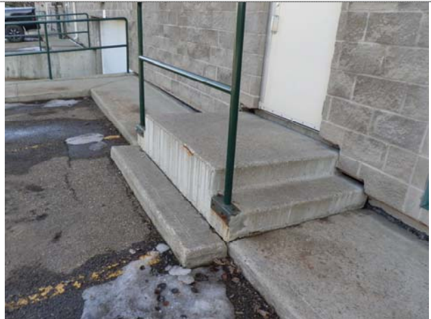
Concrete evidencing deterioration - railings rusting
