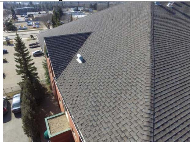
Shingle deterioration evident
