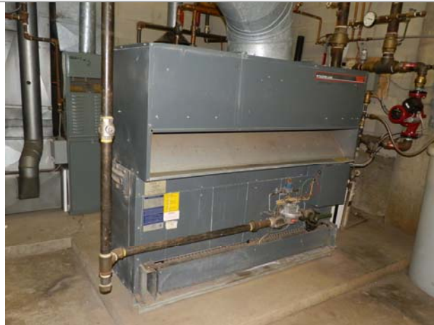
Teledyne Laars boiler M: HH 1200 IN 11K S: 1923996
