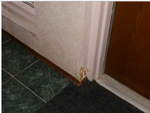
Damaged wall finish at entrance
