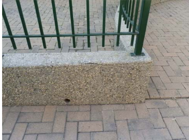
Concrete curb evidencing some minor deterioration
