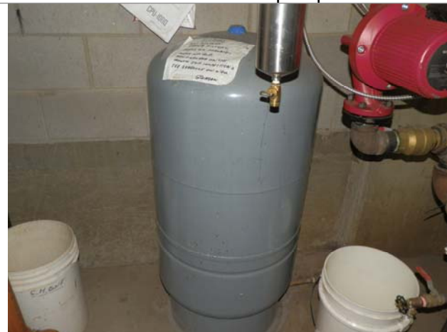
Large expansion tank
