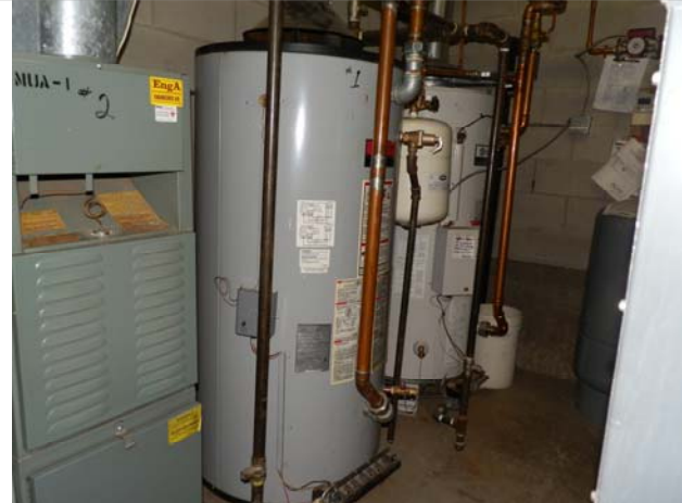
State hot water tank - 80 Gal M: SBT 80 199 NE6 DFCGA S: 02000 A.O.Smith hot water tank - 76 Gal M: BTRC199 118 S: 1337M002120
