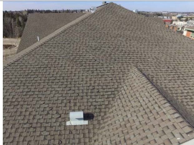
Shingle deterioration evident
