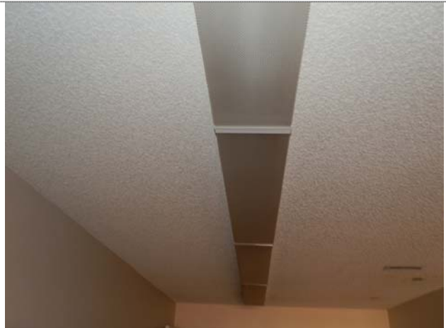
Social room florescent lighting
