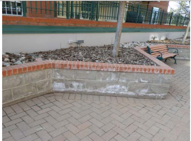
Block walls with efflorescence
