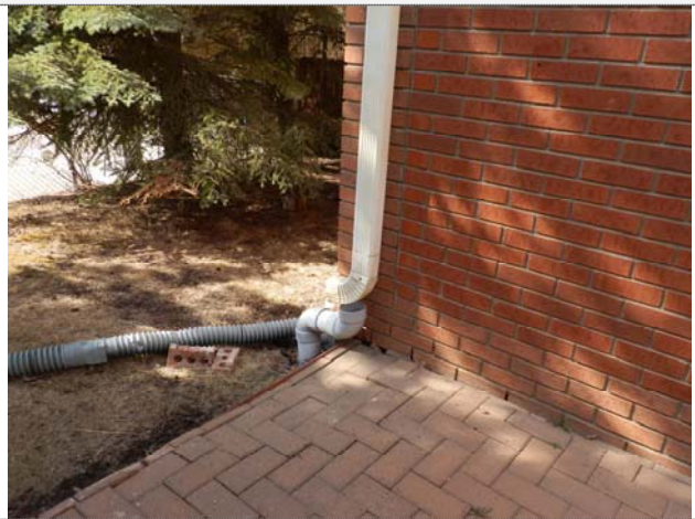
Downspout - bypassing drain - extension disconnected
