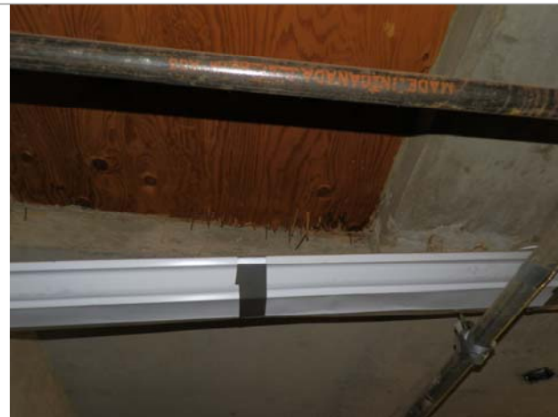
Leak in parkade ceiling
