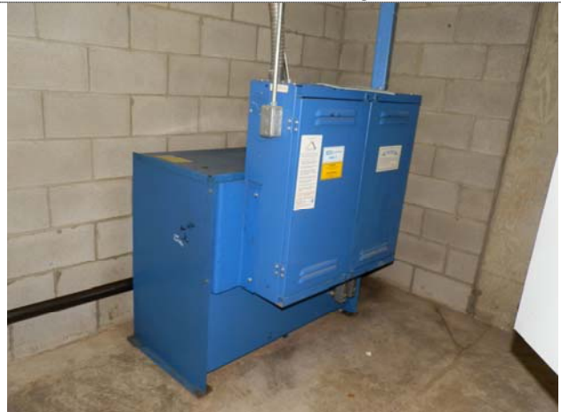
Dover elevator hydraulics M: EP-125-40 S: ED3914
