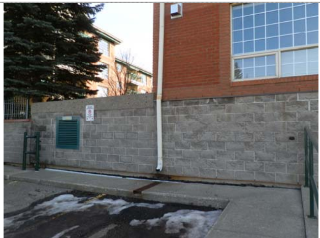
Downspout terminating onto walkway
