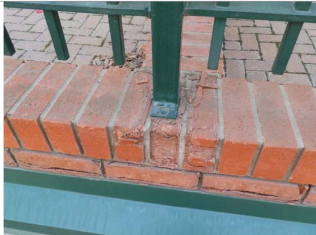
Damaged brick curbing
