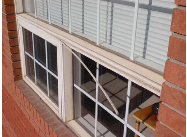
Damaged trim on window
