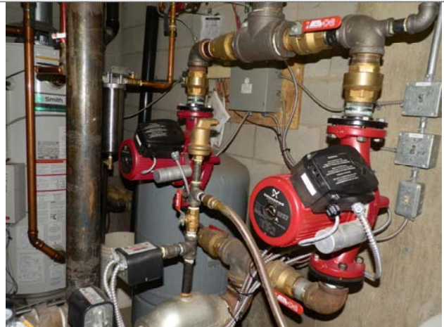
Grundfos heat/water pumps
