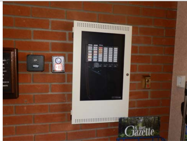
Notifier panel at entrance
